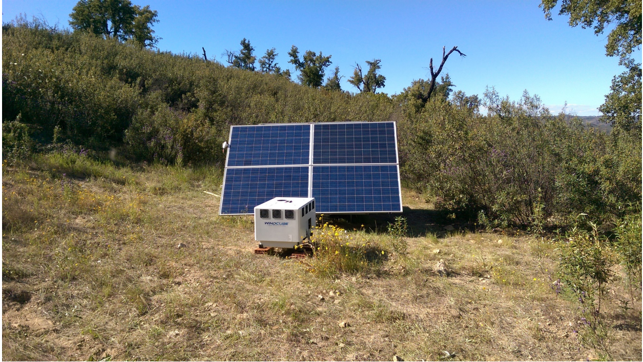
Figure 4: WC 68 at the beehive site east of the valley. This unit was operated by solar panels and a backup diesel generator provided by INEGI.
