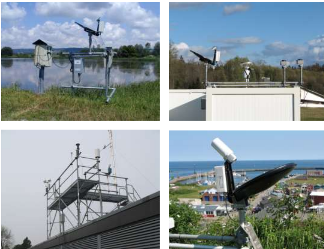
Figure 8: Examples of MRR installations
