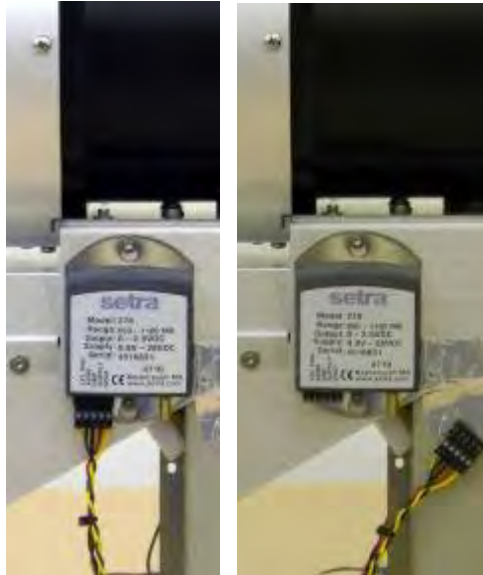
Figure G-30. Cable to Pressure Sensor, disconnected (right)
