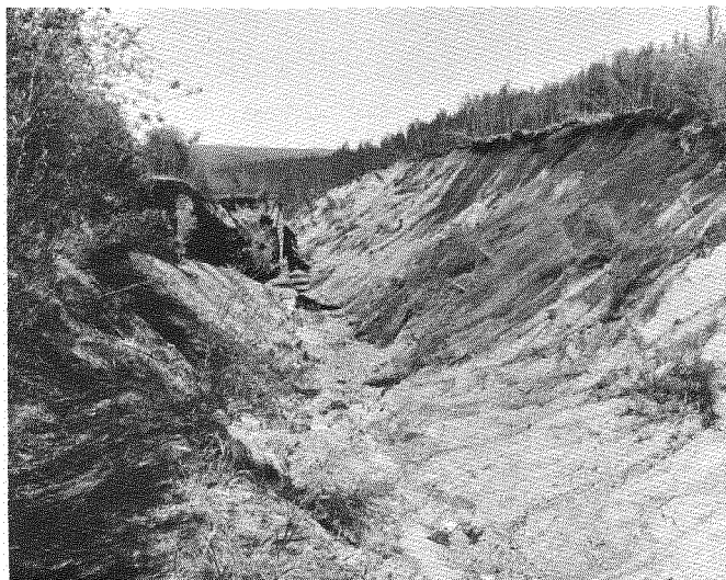
Fig. 7. View upstream in eroded spillway channel. Flat center area is at original elevation of the spillway apron
