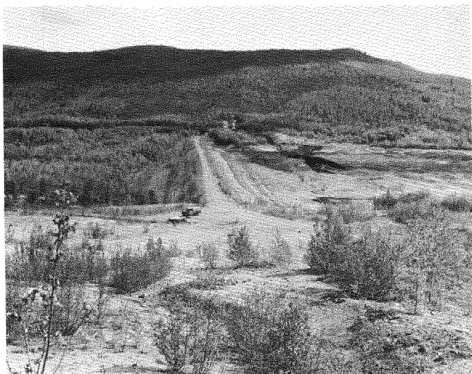
Fig. 6. General view of Hess Creek Dam from the west borrow area showing eroded spillway channel in the background
