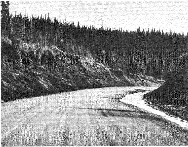
FIGURE 14 Additional slumping of backslope, 32.6 km, 28 May 1971.
