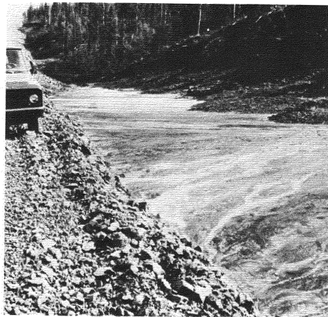
FIGURE 5 Backslope erosion into parallel ditch, 31.6 km, 26 June 1970.
