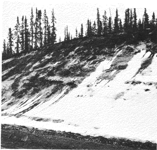
FIGURE 3 Frozen 1:1 backslope, 31.6 km, 23 April 1970.
