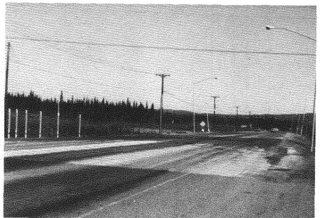
Stop 2. Note in the distance, tilting of the light standards and signs and telephone poles along both sides of the road which indicates thawing of the ice-rich permafrost with associated subsidence of the ground. (Photograph 25443 by T.L. Péwé, May 15, 1983.)
