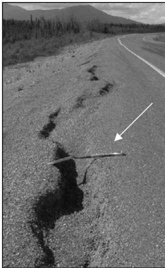
Figure 1. Longitudinal cracking along the shoulder of the Alaska Highway due to degradation of the underlying permafrost. The 1-m shovel (arrow) gives the scale.
