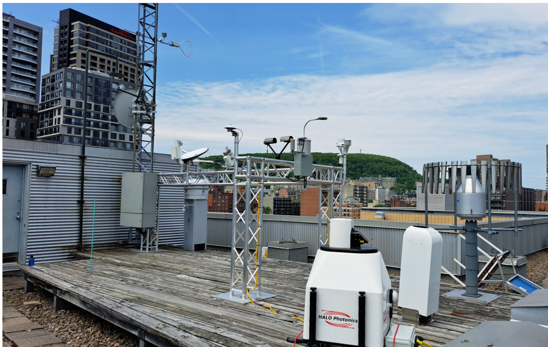
Fig. 1. Photos of the UQAM-PK weather station and the GEONOR precipitation gauge on the right.
