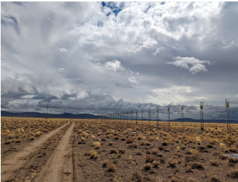
Photo 2. Image of the array and tower post Hurricane Hilary on 21 August 2023.
